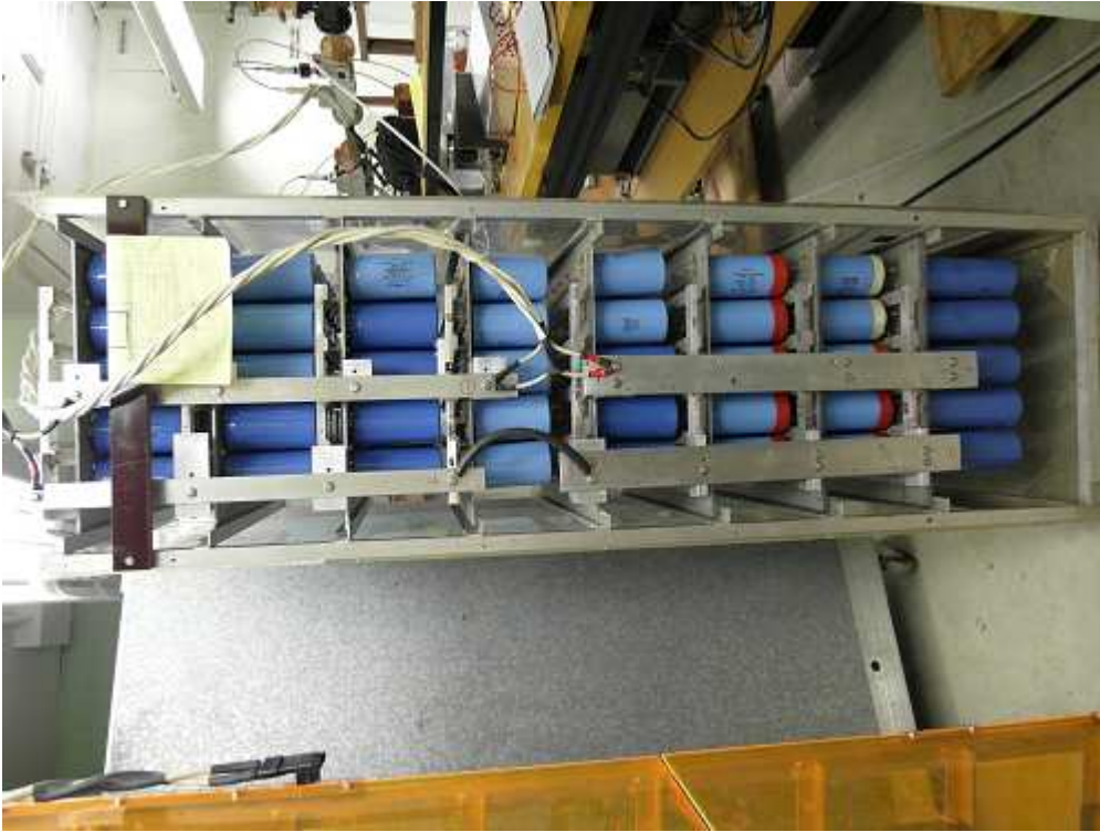
Figure 3.9 Capacitor bank bus bars.
