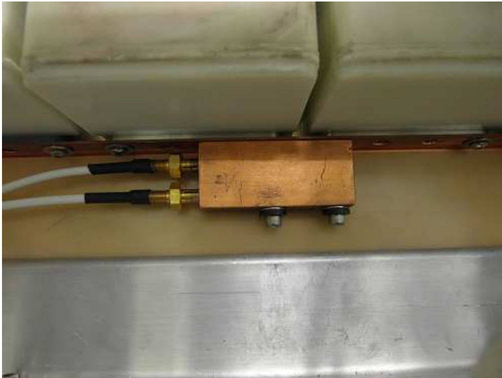
Figure 3.11 Capacitor bank interconnects.
