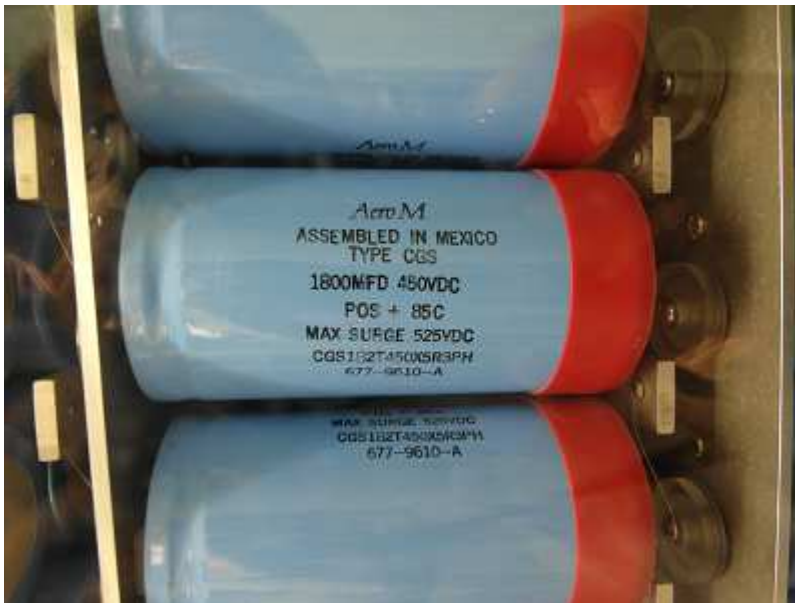
Figure 3.7 Main bank capacitors.
